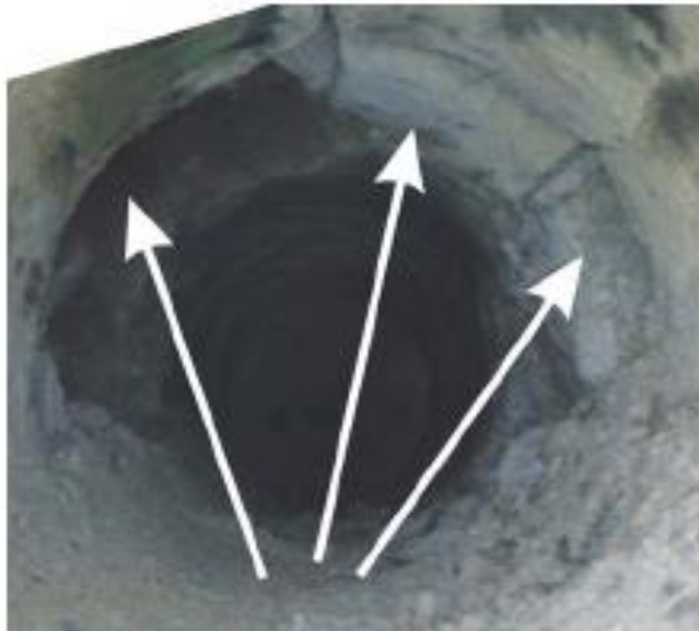
Fig. 3. The arrows mark the destruction zones of the external masonry (lining) of the pipe.
