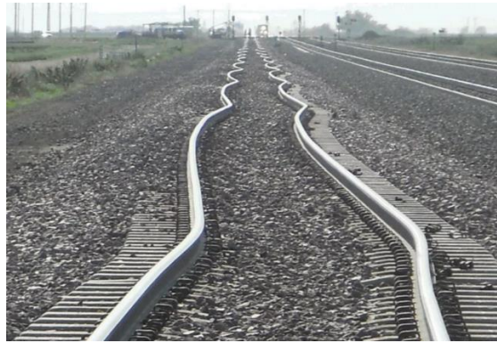
Fig. 1. Ejection of a non-jointed track in a straight section.
